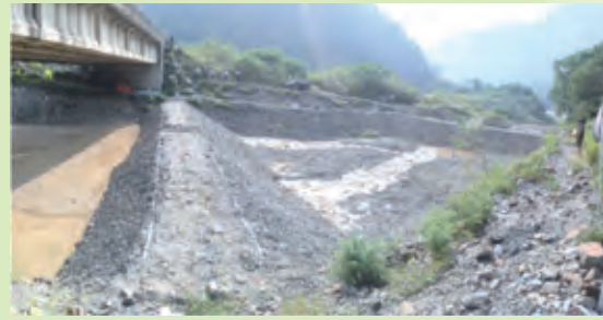
▲上圖為惠蓀林場堰塞壩潰壩試驗場域 The photo shows a landslide dam breaching test in Huisun Forest station
